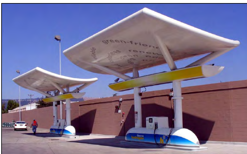
Figure 24. Hydrogen Fueling Station
