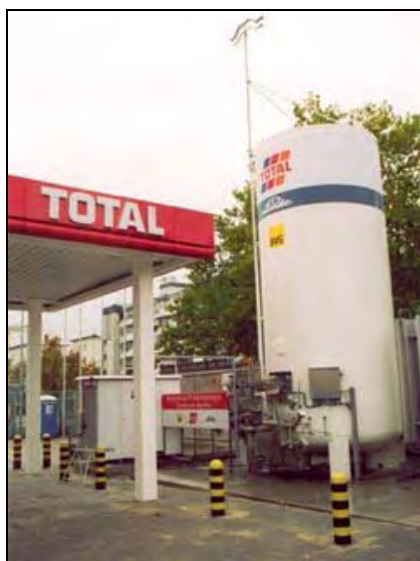
Figure 25. Liquid Hydrogen Storage Station
