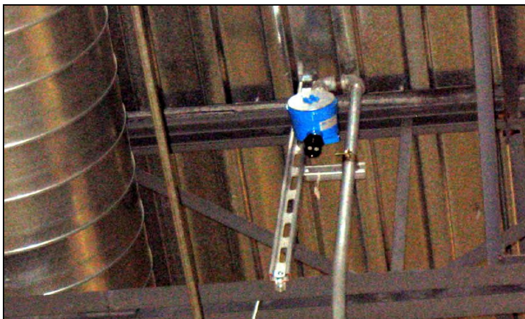
Figure 27. Hydrogen Detector Located at Ceiling Level
