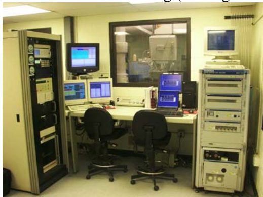
Engine Test Facility Control Room
